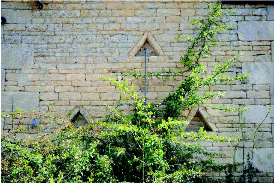
Plate 30: Detail of blocked air vents, west elevation, 3A
