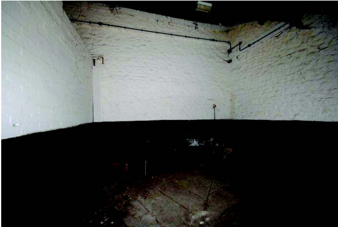
Plate 21: Northwest aspect, northern stable, 2B, showing original walls of 2A and 2B
